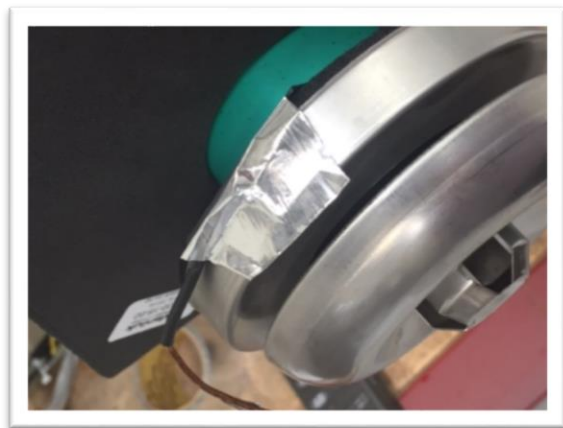
Figure 7: Location of thermocouple on the mushroom flue adjacent to likely cladding material
